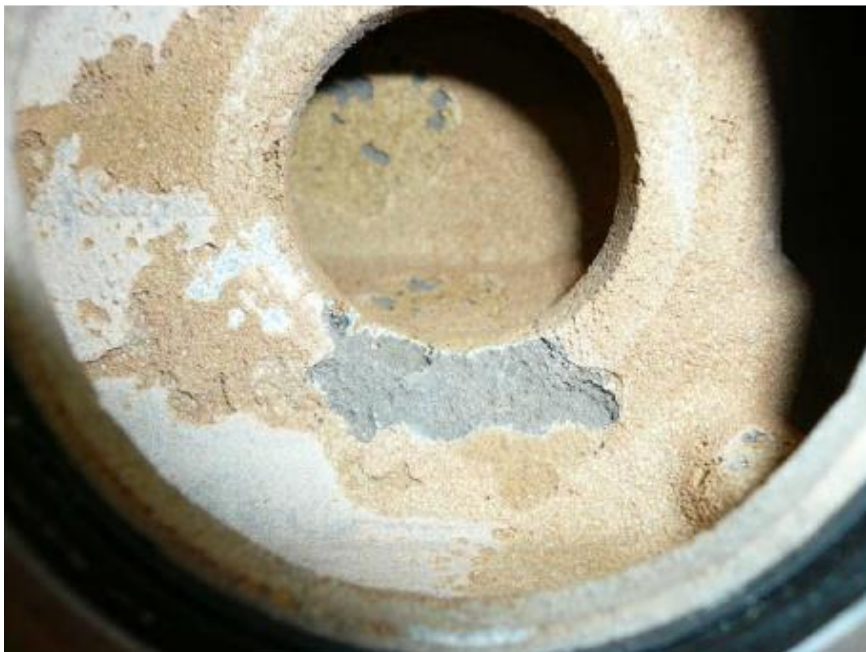
A 4 Aluminium thermostat cover, corroded
